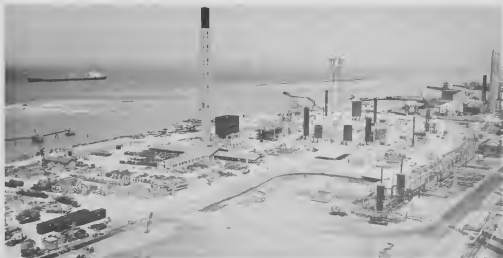
Construction progressing on Hydrodesulfurization units June 1. Construccion progresando ariba Planta Desulfurador Juni 1.
